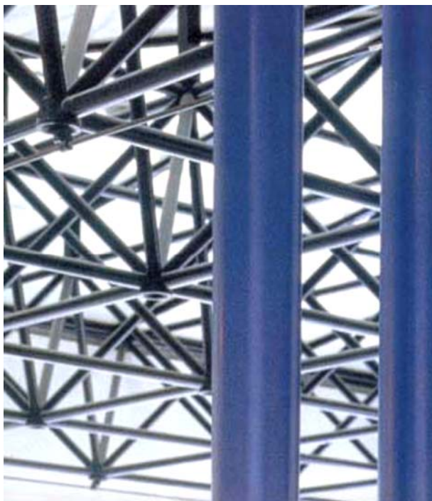
9.25 Application of the 'technical plant stem': lightweight load-carrying roof substructure (courtesy Exel-Oy).
